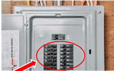
Basement auxilliary panel needs proper labeling.
