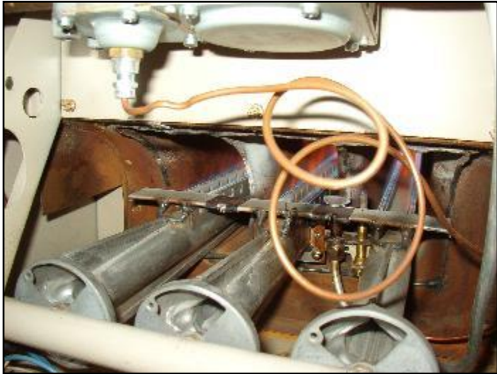
9. Rust at bottom of heat exchanger
