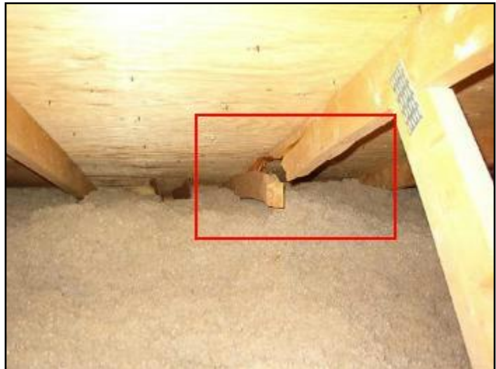
6. Top chord of truss is broken
