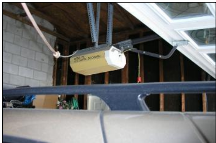
17. Extension cord for west garage door opener
