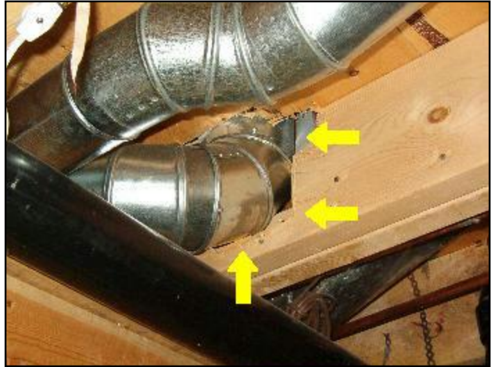
5. Joists are notched and weakened
