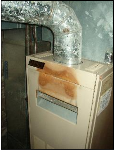
10. Evidence of furnace backdrafting
