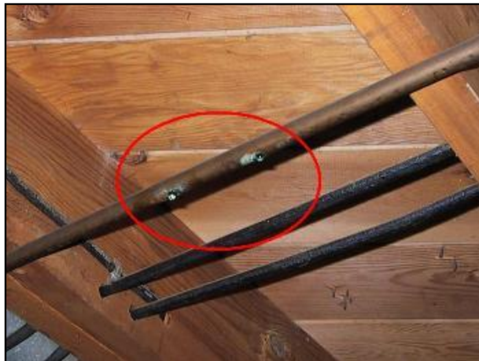
13. Leaking copper supply pipe
