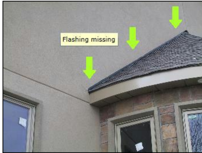
1. No kickout flashing at roof/sidewall junction
