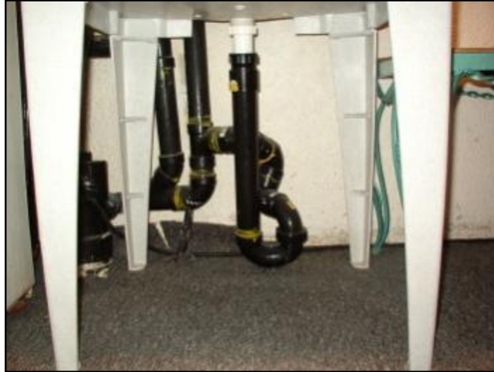
14. Poor trap arrangement
