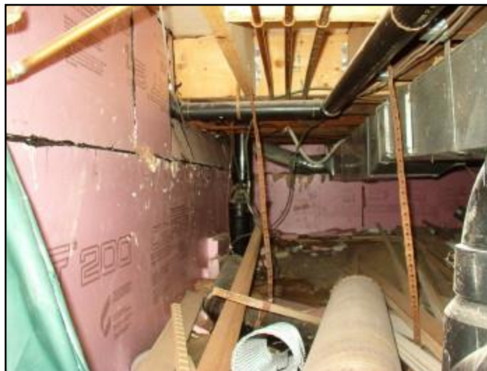
12. Exposed polystyrene insulation is fire hazard
