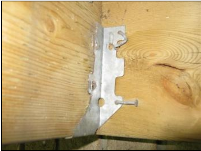
4. Poor end bearing, joist hanger connections
