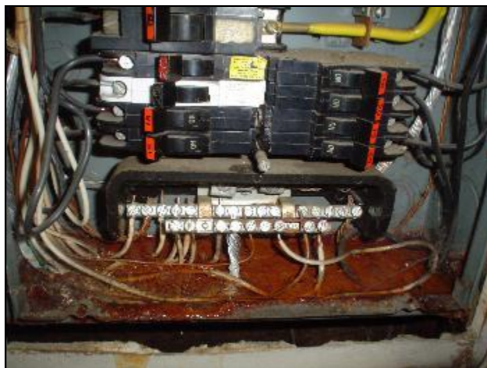
7. Water and rust in bottom of panel
