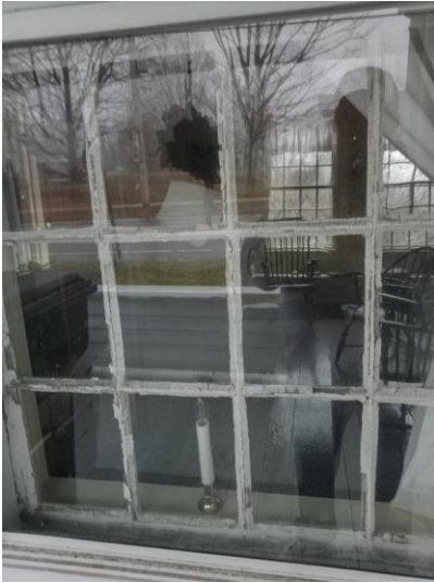
An example of original 12 over 12 window that needs to be re-glazed
