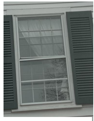
An example of present storm windows in disrepair.
