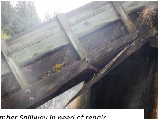
Timber Spillway in need of repair.
