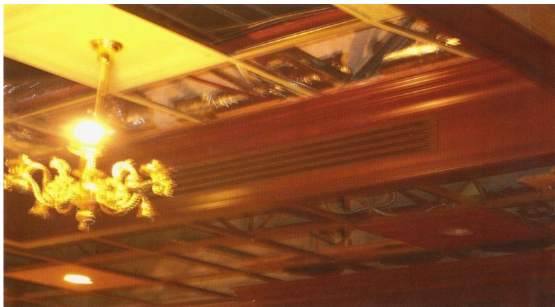
Shows the linear diffuser installed in the beautiful woodwork
