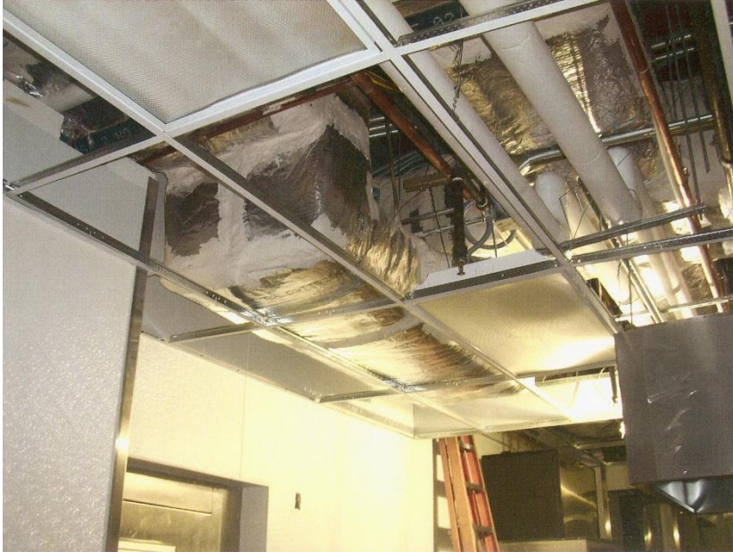
Shows congestion above the ceiling
