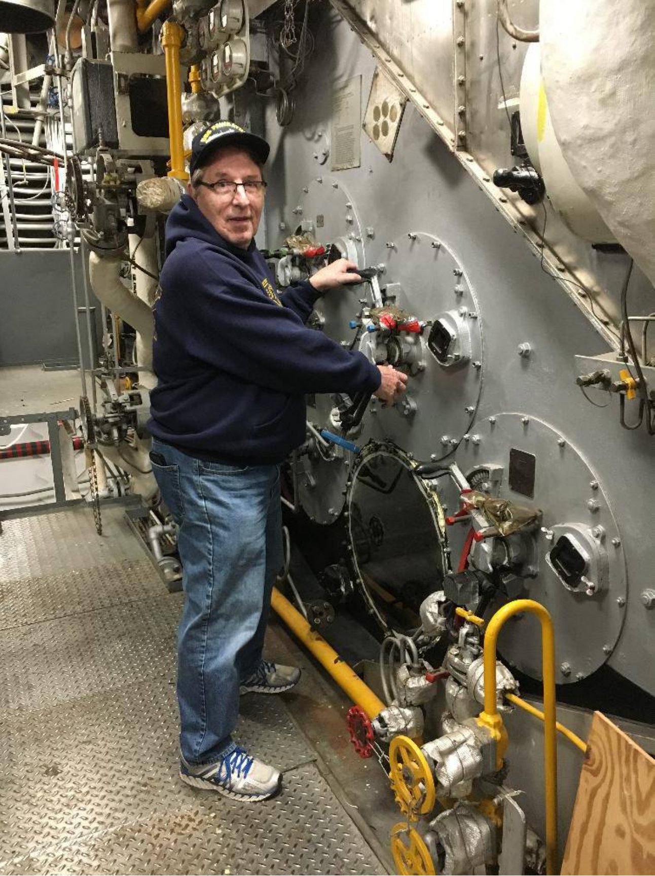
Charlie at a boiler getting ready to load a burner.
