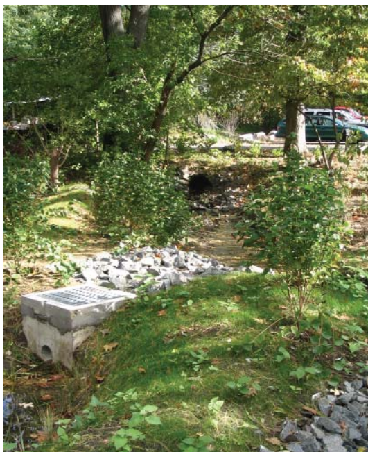
Stormwater treatment, Westchester
