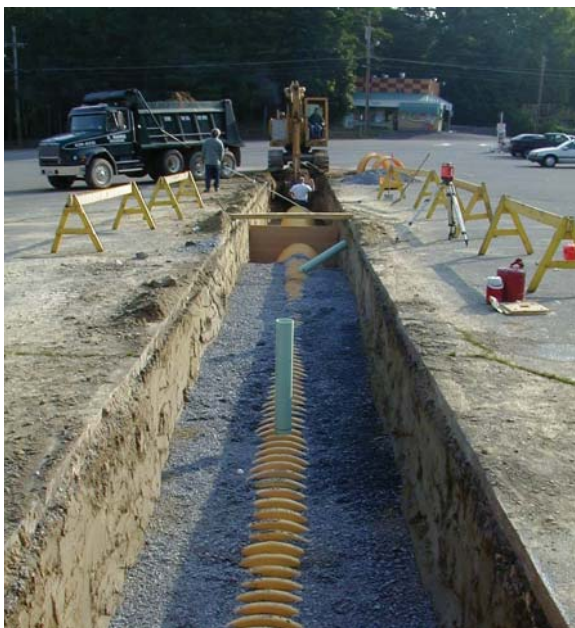
Stormwater treatment installation
