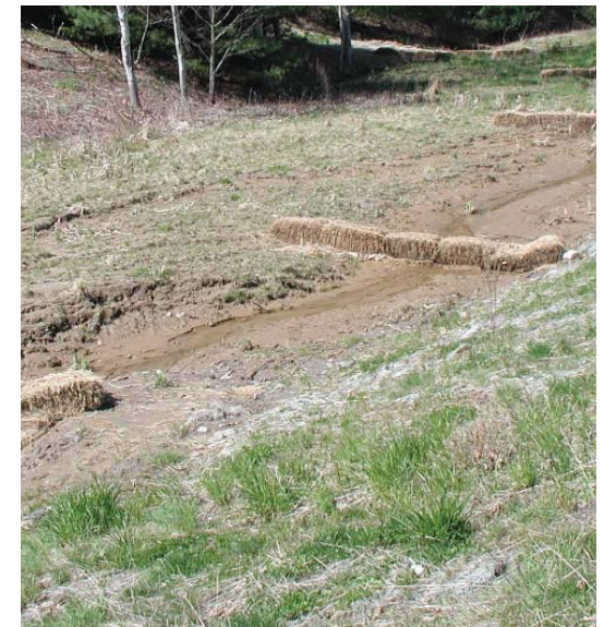
Improper use of control measures
