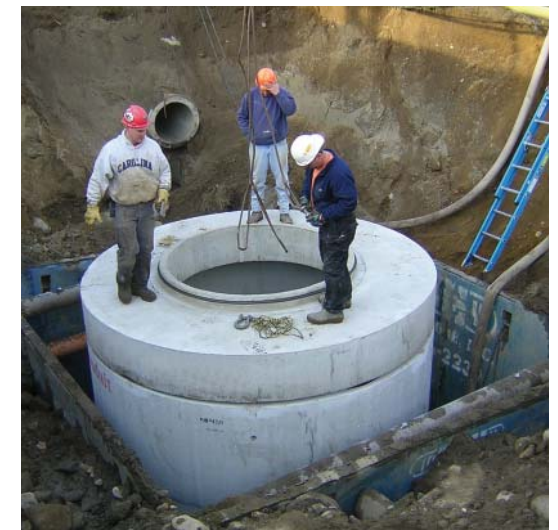
Stormwater treatment installation, Lake George
