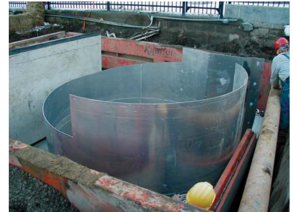
Stormwater treatment system
