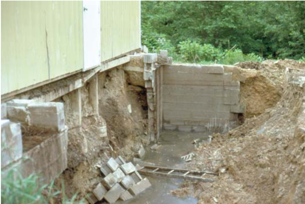
Foundation failure caused by excess water. (Photo by Pennsylvania NRCS.)
