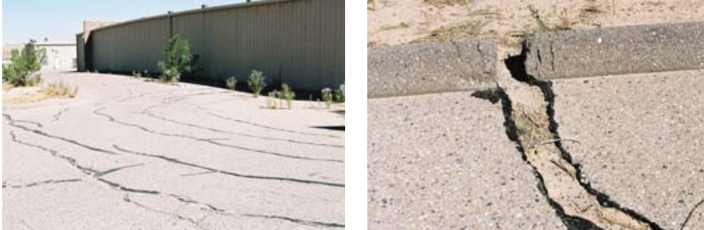
Concentric cracks caused by soil collapse near abandoned buildings in New Mexico. (NRCS photos.)
