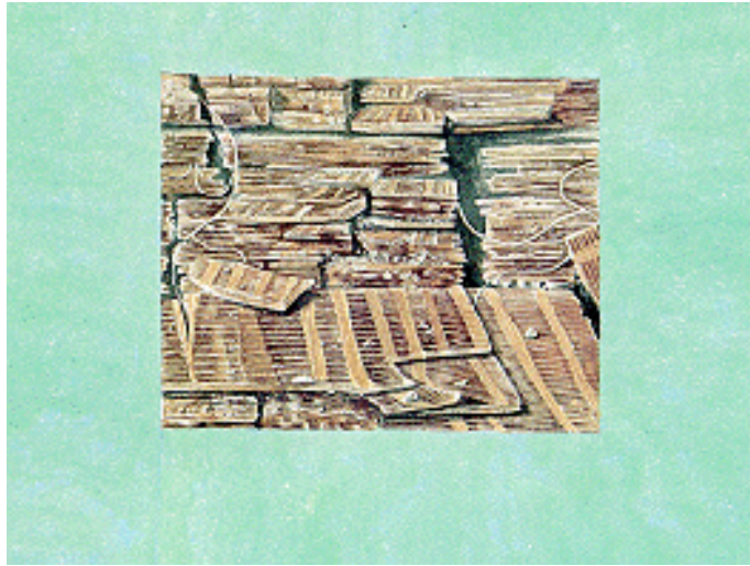
Figure 95 Closeup of brown rot in pine
