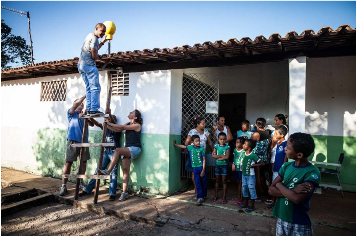
Figure 1-4 Early Loon fixed wireless service. Installing terminals on roof of school in Agua Fria, Brazil.
