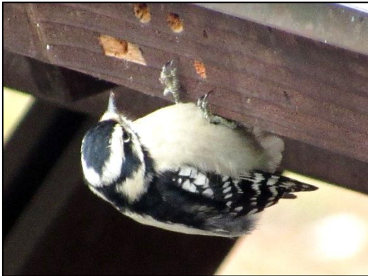
Downy Woodpecker causing damage in Courtyard
